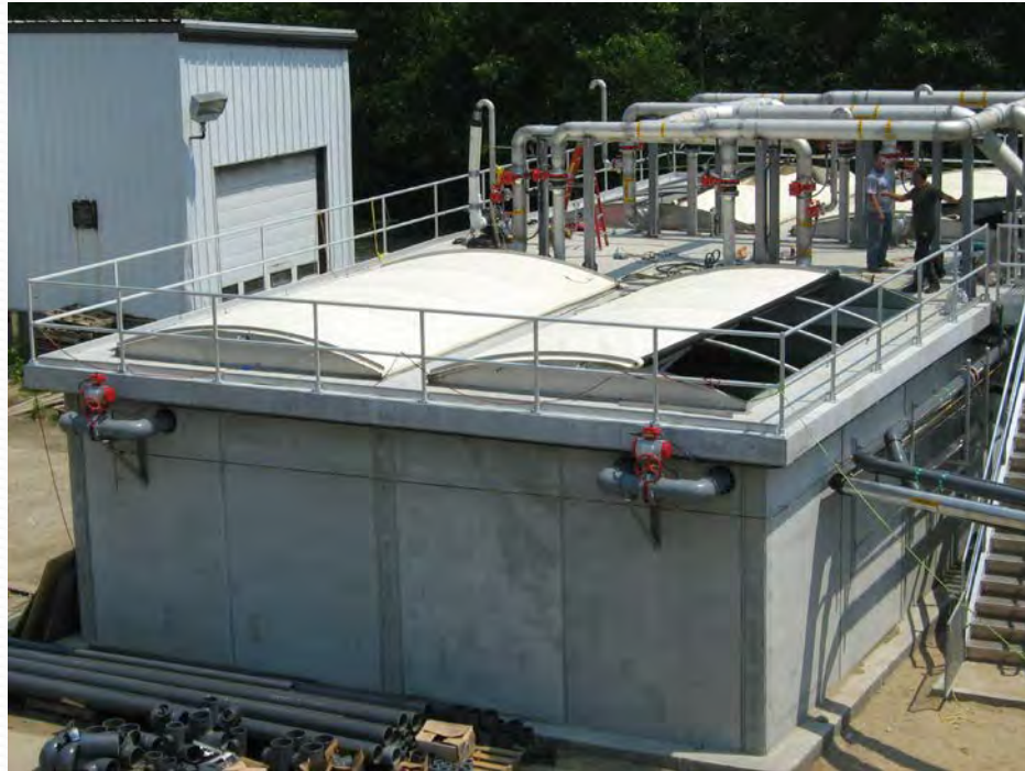
AnMBR ® system. Photo courtesy of Evoqua.
